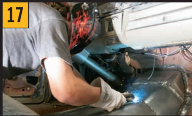
17 The three pieces of sheet metal were stitch welded into place, which marked the completion of the new transmission tunnel.
